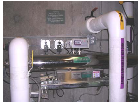
Outflow valves for tank
